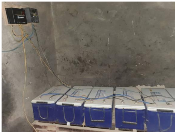
Fig. 7: The solar system installed in the green building (Field Survey, 2020).
